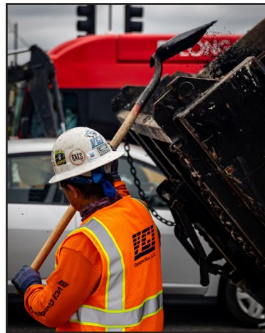
Richard H. Grant | Signal Tribune A construction worker tosses unused asphalt while repairing part of the intersection of Pacific Coast Highway and Cherry Boulevard on May 9, 2023.
