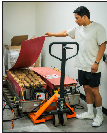
Richard H. Grant | Signal Tribune An employee at ReJoule inspects extra large lithium-ion battery packs that will be tested in the high voltage area of their lab on Oct. 4, 2023.
