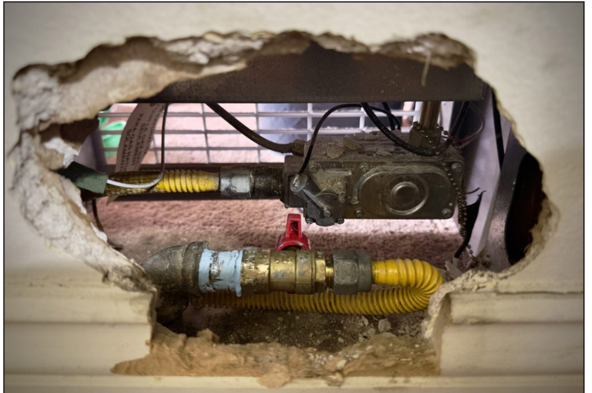
Richard H. Grant | Signal Tribune An exposed natural gas line connected to a wall heater is seen through a hole in the wall of an apartment in Long Beach on Feb. 2, 2023.
