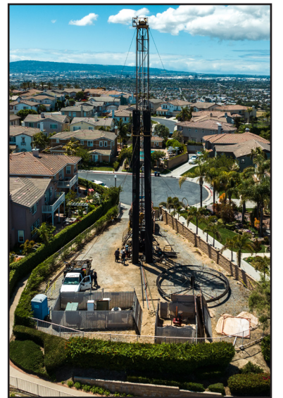
Richard H. Grant | Signal Tribune Workers move around an oil well at the top of Signal Hill inside of the neighborhood on May 2, 2023.
