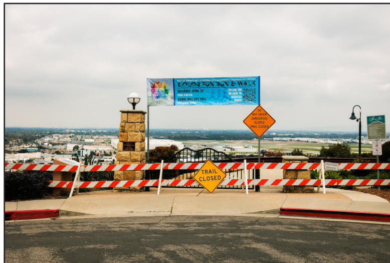
Richard H. Grant | Signal Tribune Signs block passage onto the Panorama Promenade Park Trail in Signal Hill on Feb. 27, 2024 due to land erosion caused by storms.
