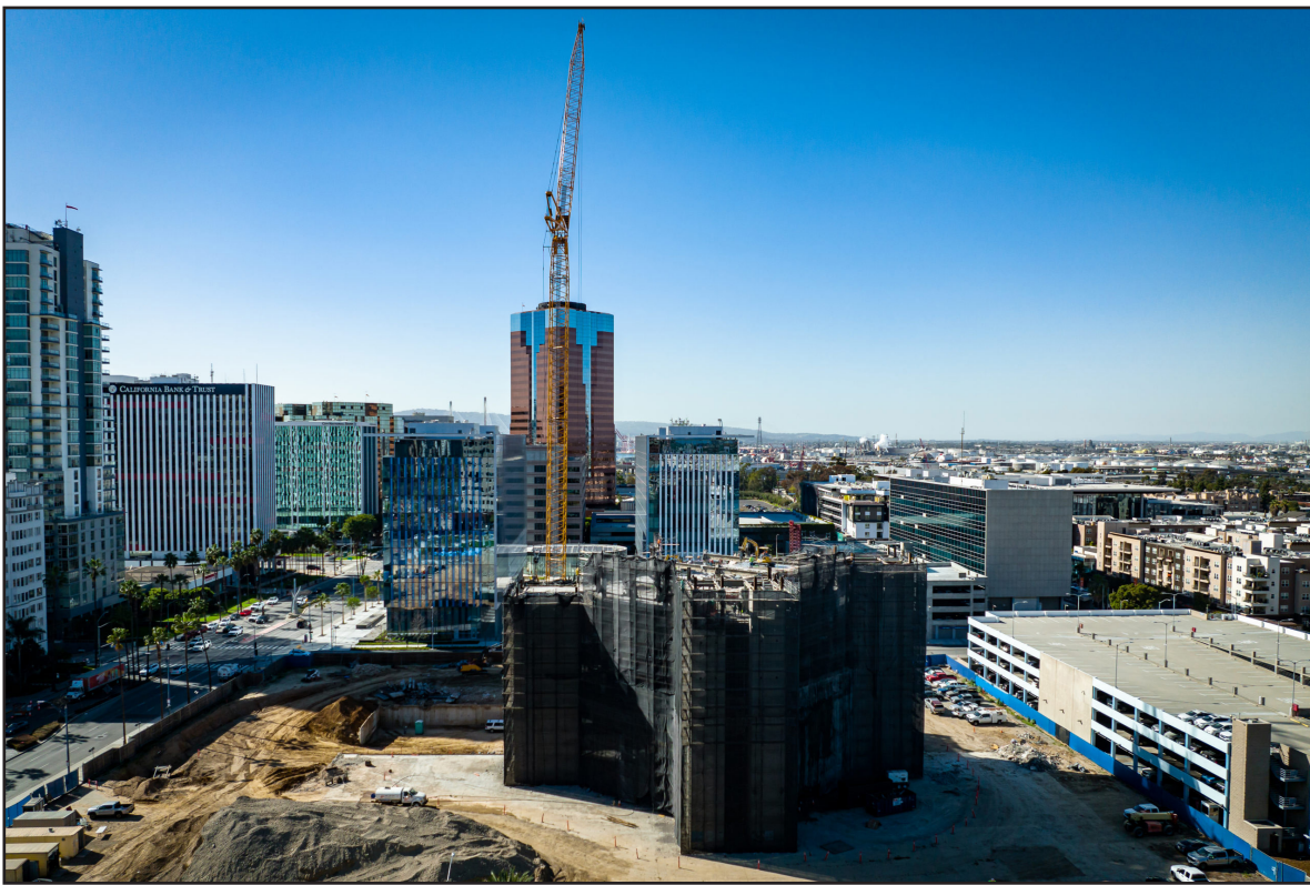
Richard H. Grant | Signal Tribune Workers continue to tear down the remains of the previous Long Beach Civic Center on Feb. 2, 2022.
