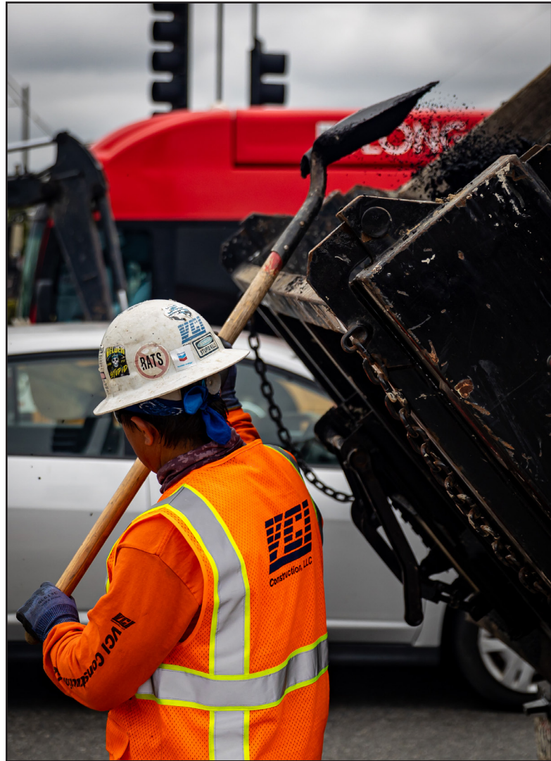
Richard H. Grant | Signal Tribune A construction worker with VCI Construction uses a shovel to toss the unused asphalt back into a truck while repairing part of the intersection of Pacific Coast Highway and Cherry Boulevard in Long Beach on May 9, 2023.
