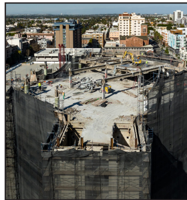
Richard H. Grant | Signal Tribune Workers continue to tear down the remains of the previous Long Beach Civic Center on Feb. 2, 2022.
