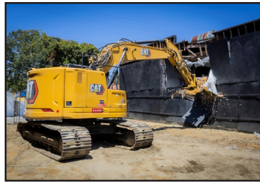
Courtesy of the City of Long Beach City officials and representatives from Vincor Construction, Inc. commemorate the demolition of the commercial properties located at 5641-5649 Atlantic Ave. on July 30, 2025.
